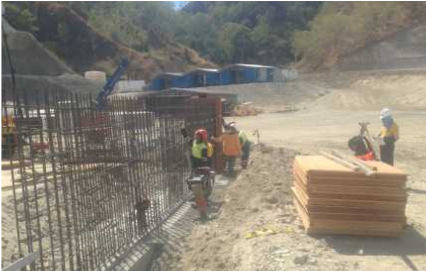
Image 3 – Formwork for concrete pour at the SX area of the 25kt SX-EW plant
