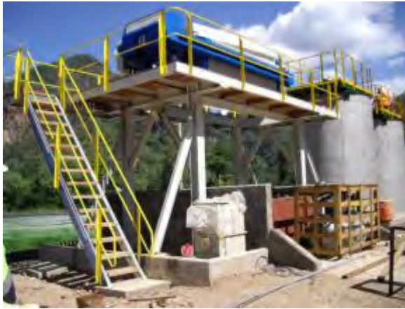
Figure 5. Filter press and neutralisation plant
