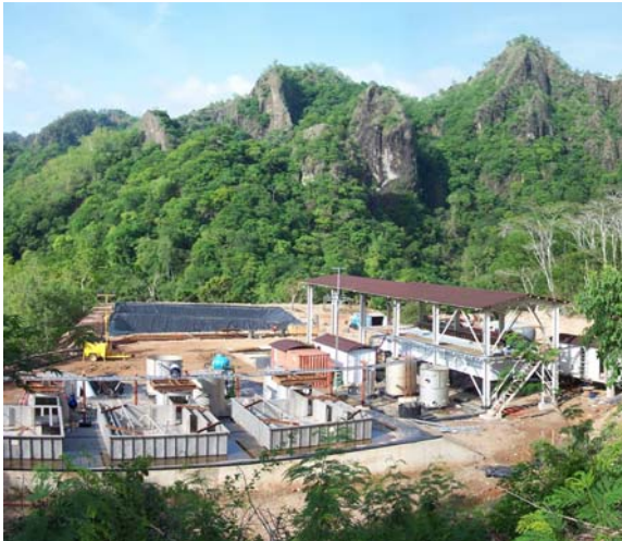
The Wetar Demonstration Project SX-EW plant, December 2008.
