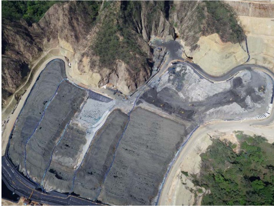
Image 2 – Leach pads KK01 to KK06 with final portion of Pad KK03 being re-lined
