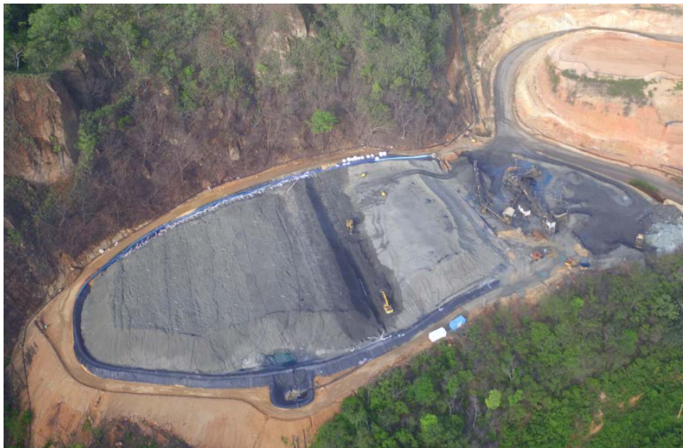
Image 3 – Leach pad DP07 during re-mining phase. Production increased 5-fold as a result of the improvements made
