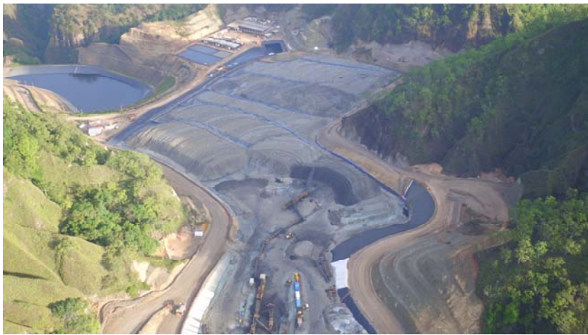
Image 5 – Aerial view of the 25,000 t.p.a. SX-EW looking across the KKV Heap Leach Pad
