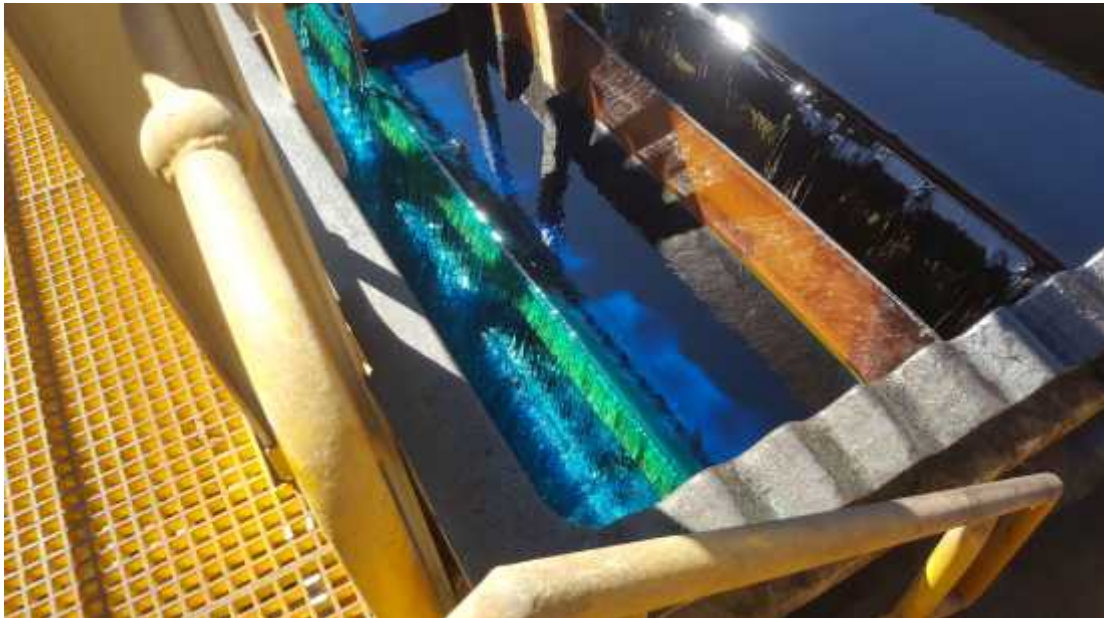
Figure 3: Electrolyte solution flowing out of the solvent extraction settlers to the electrowinning circuit
