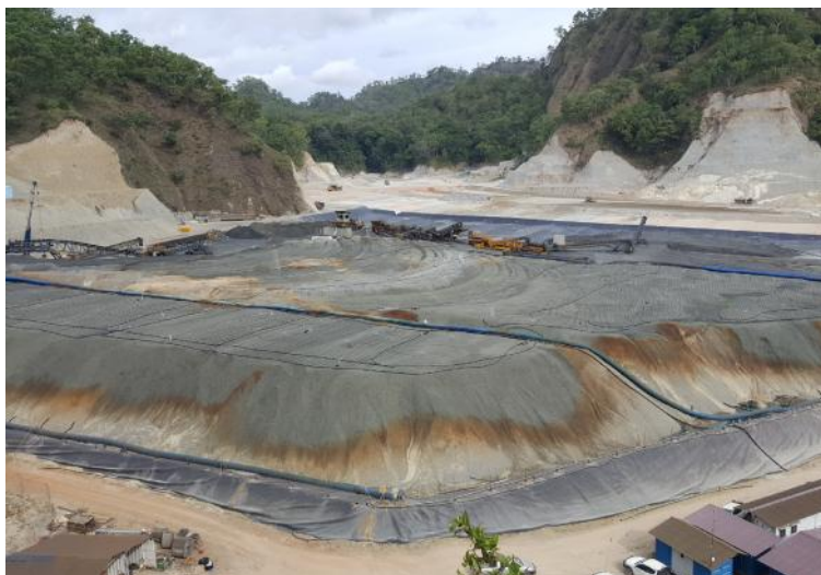
Image 3 – Kali Kuning Valley Leach Pad
