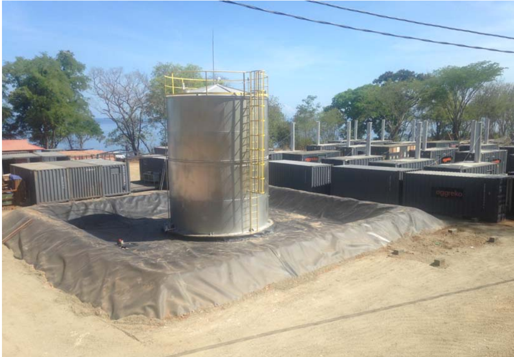
Image 5 – Power station and fuel tank
