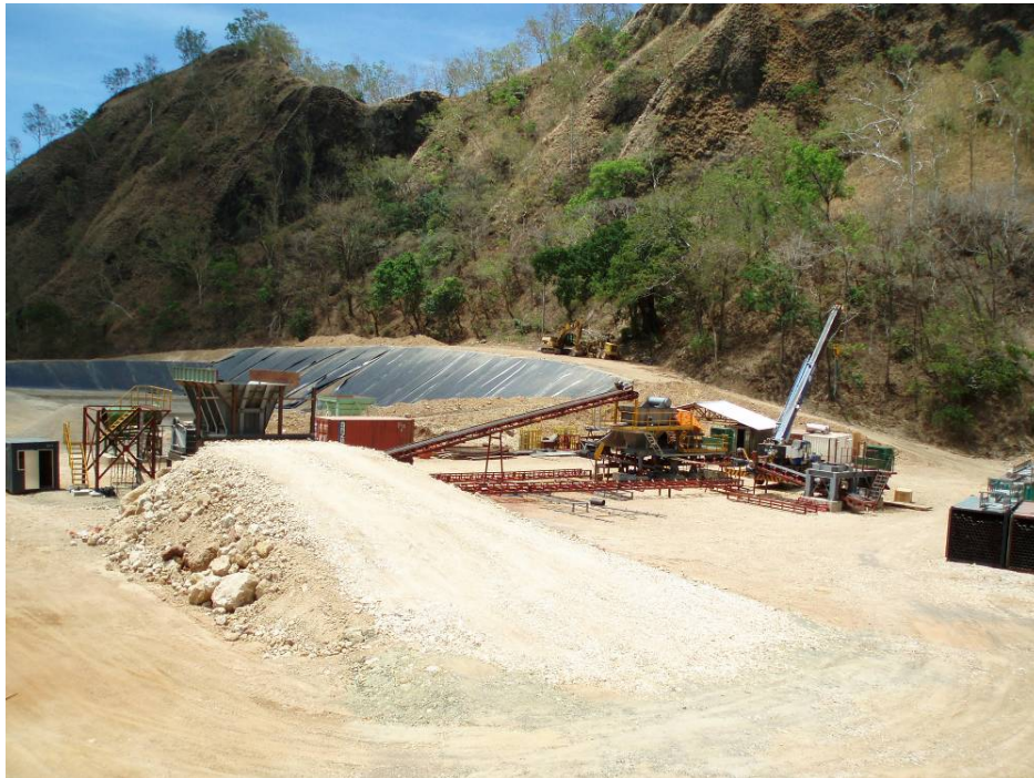
Crusher and Leach Pad at Wetar Demonstration Plant
