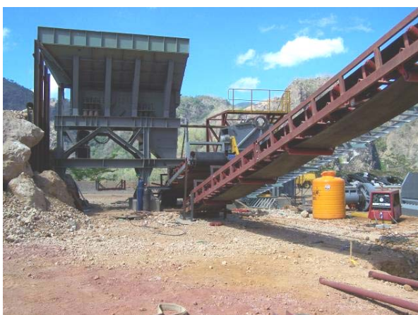
Primary Crusher & Conveyors
