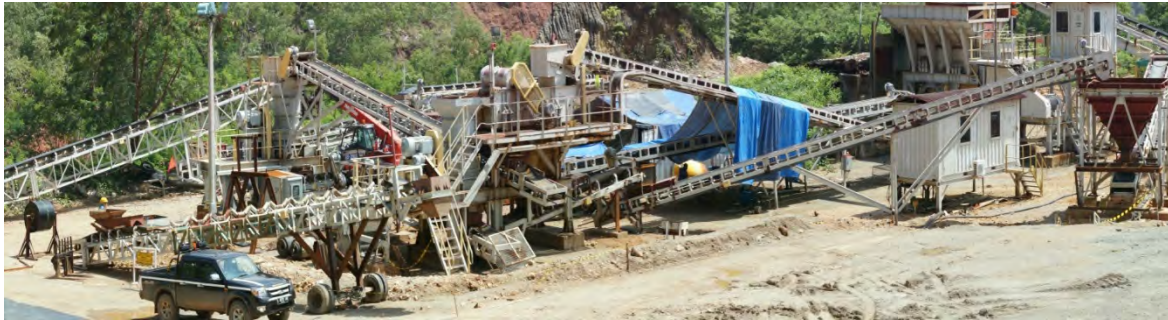
Photograph above shows the refurbished crushing plant awaiting the commencement of stacking operations.
