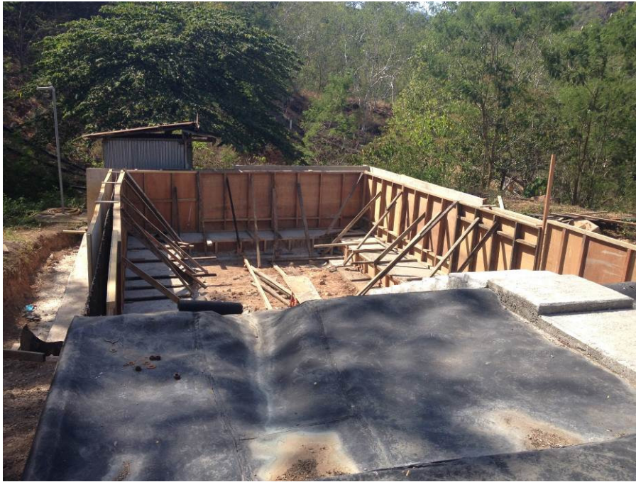
Formwork for new wash settler. The wash settler purifies and concentrates the leach solution after it comes off the heaps and before it is piped into the electro-winning plant
