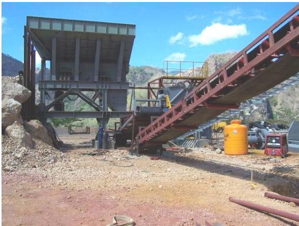
Primary Crusher & Conveyors
