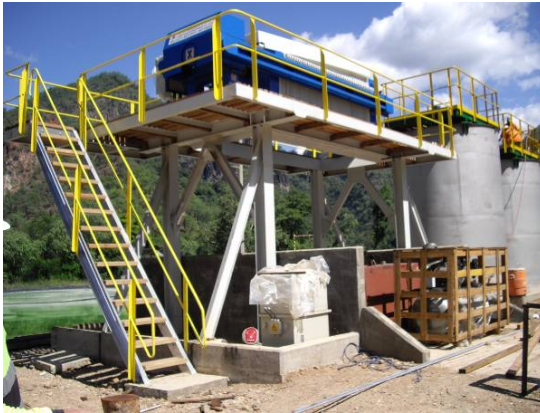
Fig 2: Filter Press and neutralisation Plant
